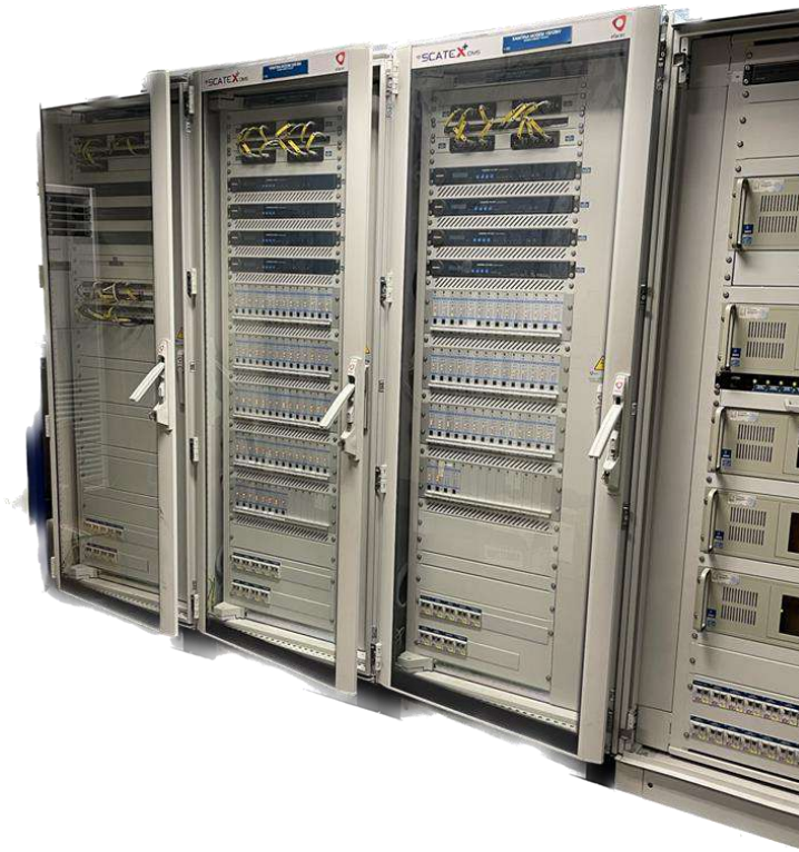
Figure 16. Greek Demo – AMI Infrastructure.
